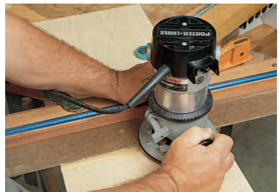
The dados for the headboard's straightforward joinery are plowed while the sides and dividers are still rectangular. The angled front edges are laid out and cut next.
