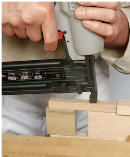
Figure 14: The hidden parts of the joint can be reinforced with staples. A dowel is better.
